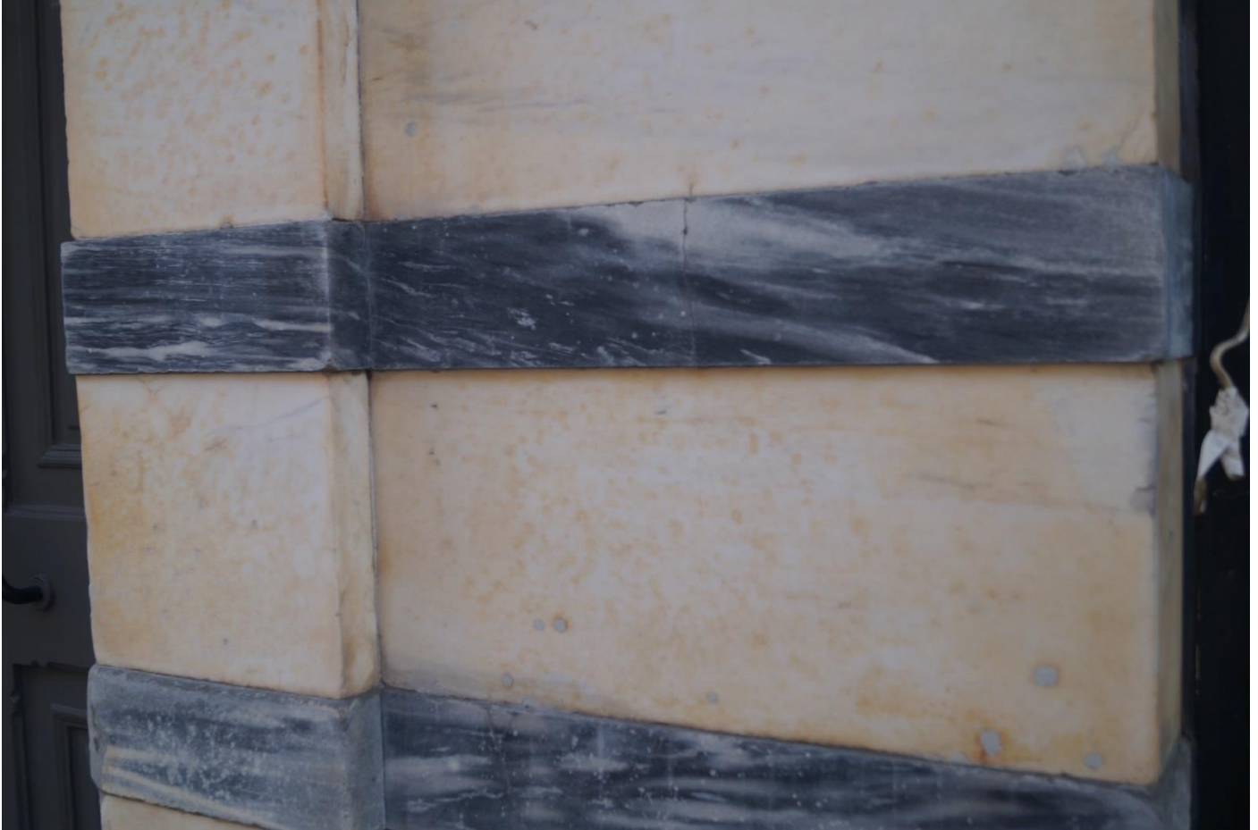
Honed slabs of Furuli marble and Antique marble in building in Oslo, late 19 th Century. Note rusty spots due to iron content in dolomite.
